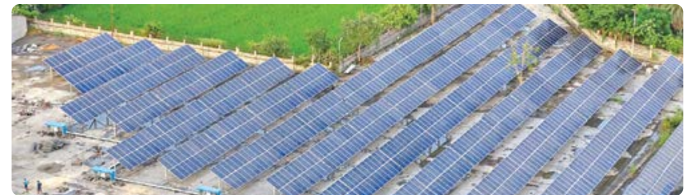
SCL solar plant at Panipat
